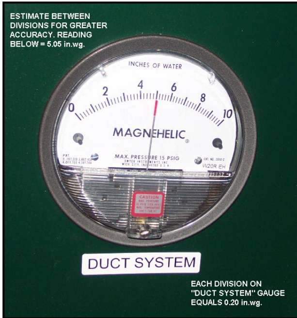
Figure 15 – Duct System Gauge Pressure Reading
